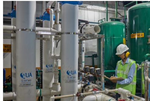
STP Plant with Ultra-filtration
